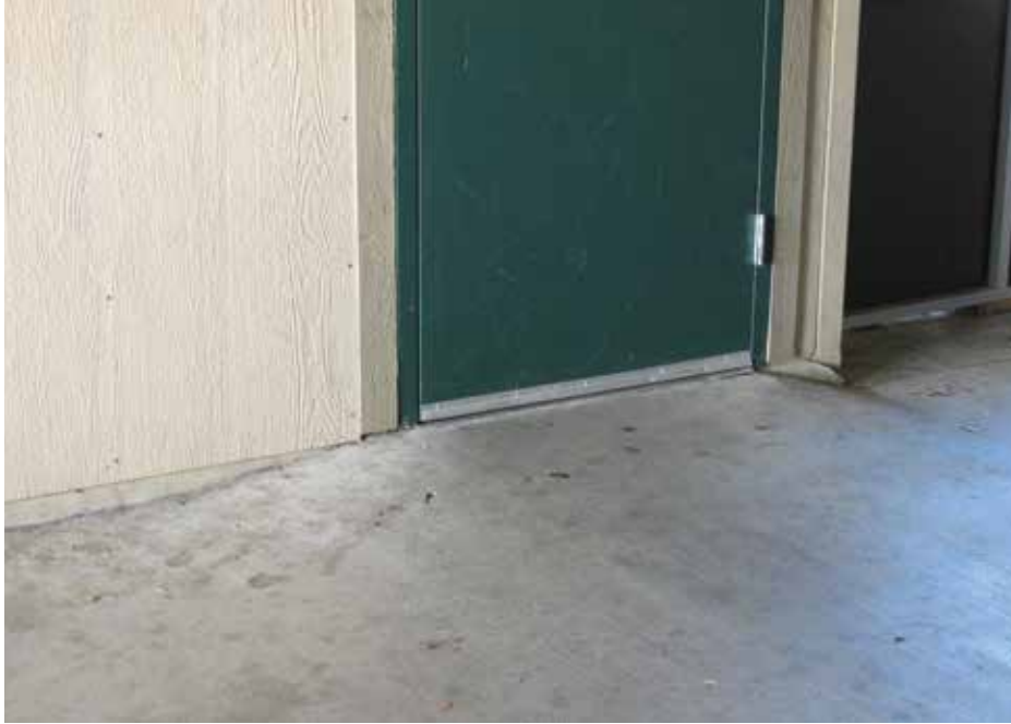
Existing exterior door with no strike-side clearance level-landing and non-compliant cross-slope.
